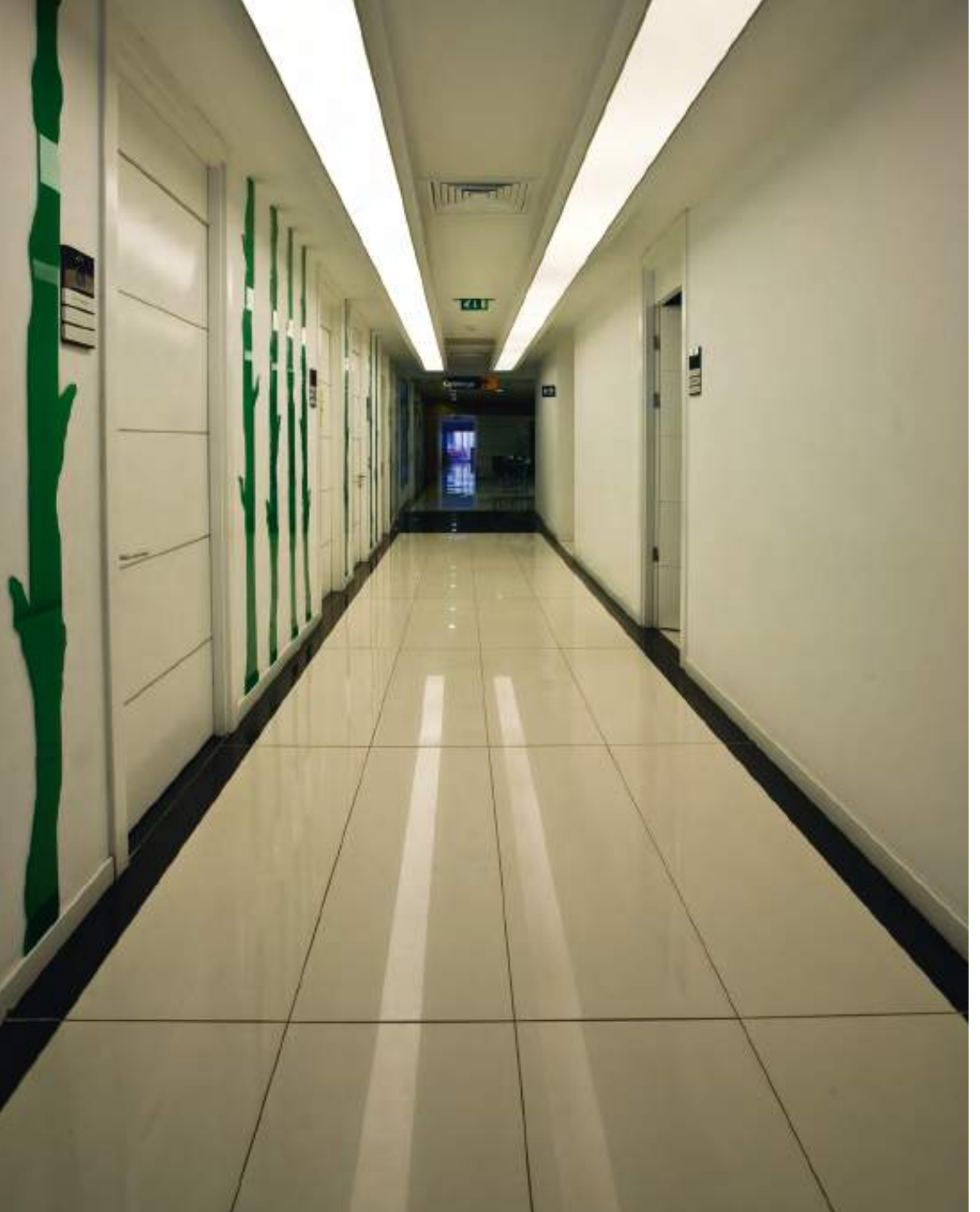
Kent Hastanesi, Alsancak / İzmir — Zemin Uygulaması — Kalesinterflex 5mm Fit Beyaz Kent Hospital, Alsancak / İzmir — Floor Application — Kalesinterflex 5mm Fit White Mimar: RSG — Architect: RSG
