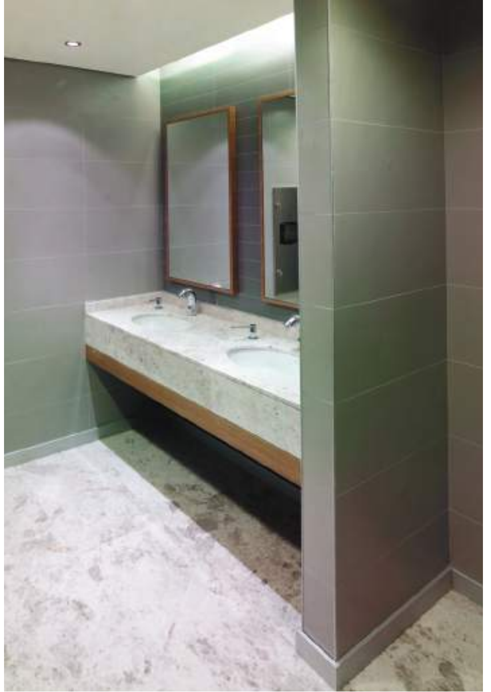
Nida İş Merkezi / İstanbul — Duvar Uygulaması — Kalesinterflex 3mm Fit Çimento Gri Nida Business Center / İstanbul — Wall Application — Kalesinterflex 3mm Fit Cement Grey Mimar: MDARCH — Architect: MDARCH
